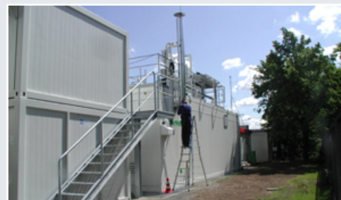
New LPG reformer ready for action at Heerstrasse, Berlin.
